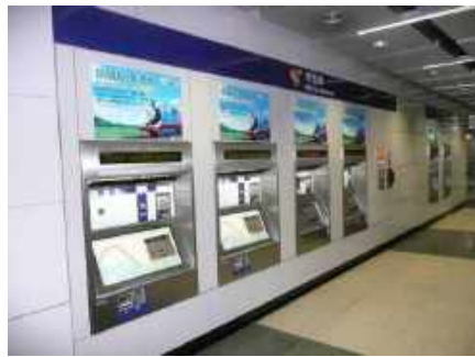
MTR Wall mounted TVM with maintenance corridor in the back – Hong Kong
