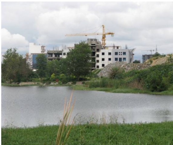
Picture 2a: Construction work being carried out near the east bank of the lake.
