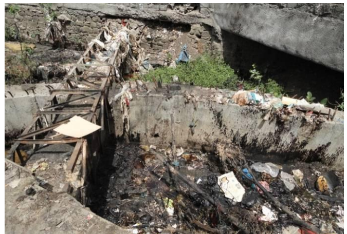
Plate 4-2: Wrong practice of disposal of waste into drains
