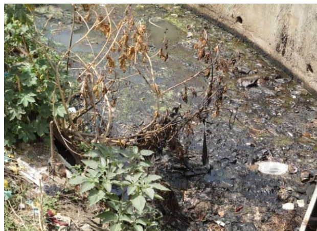
Plate 4-8: Choked drain due to disposal of waste
