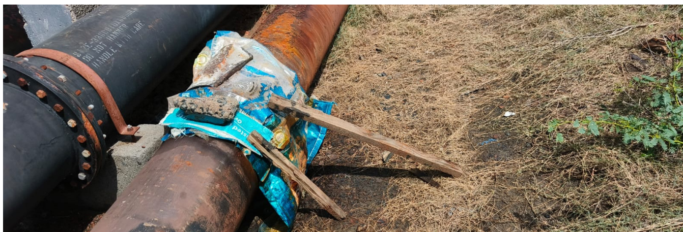
Figure 9: Ash pipeline leak from a n unreplaced (old) pipeline. Photo dated 13 July 2025
