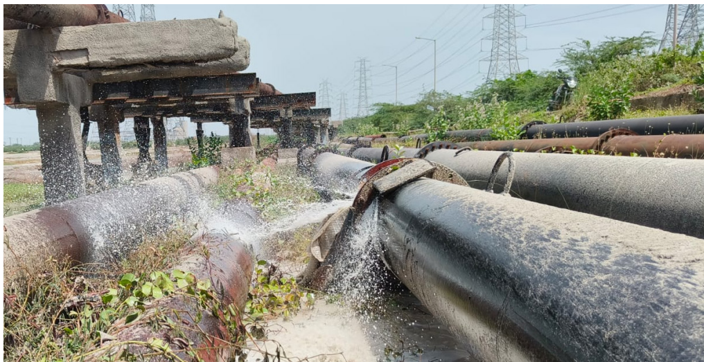
Figure 8: Ash pipeline leak from a replaced (new) pipeline. Photo dated 13 July 2025
