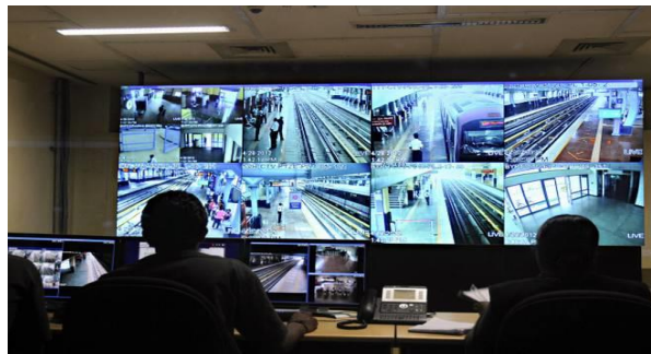
Figure 15.3 Station Control Rooms
