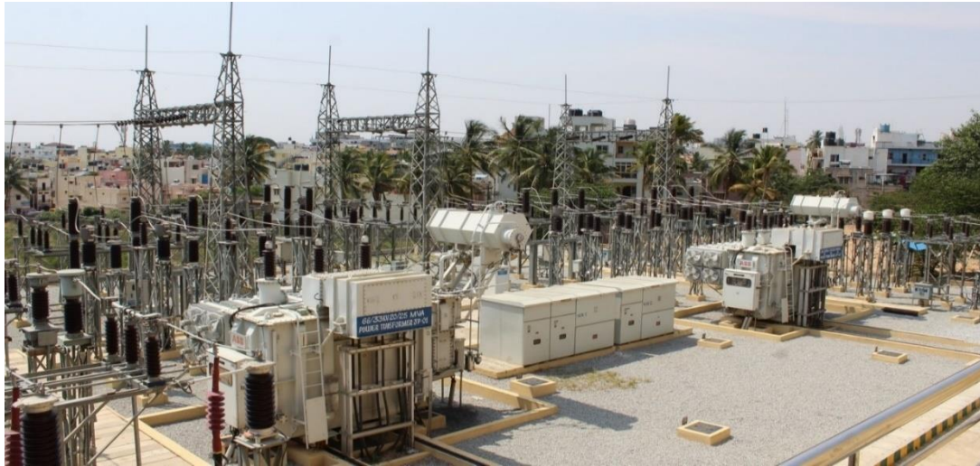
Figure 12.1 Typical High Voltage Receiving Sub-Station
