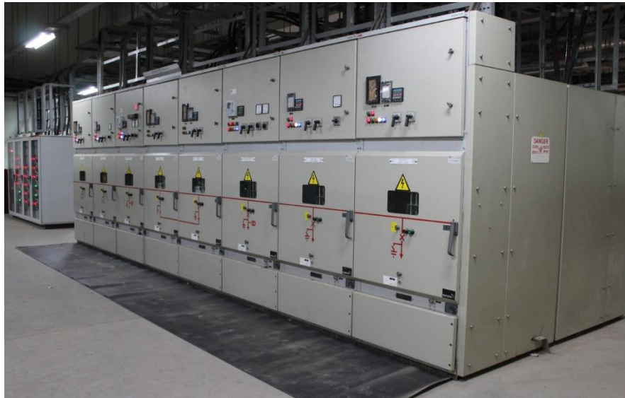
Figure 12.4 Typical Indoor Auxiliary Sub-station
