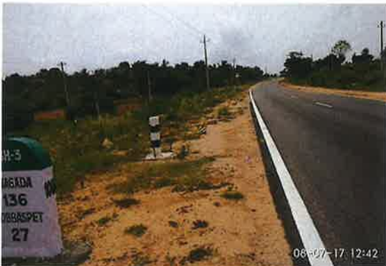
Existing road condition of SH-3 (Km 27.500)
