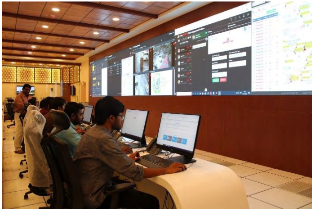
FIGURE 5.3: INTEGRATED COMMAND AND CONTROL CENTER (ICCC) ESTABLISHED BY GCC
