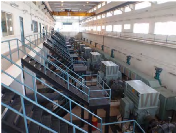
Photo 3.2.3 TK Halli Pump Station
