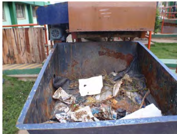
Photo 4.3.3 Container for Screenings
