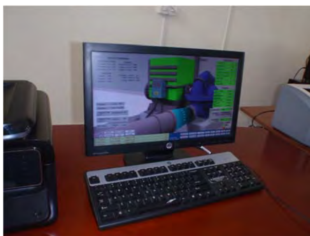
Photo 3.2.5 SCADA in Tataguni PS (Stage IV Phase 2)
