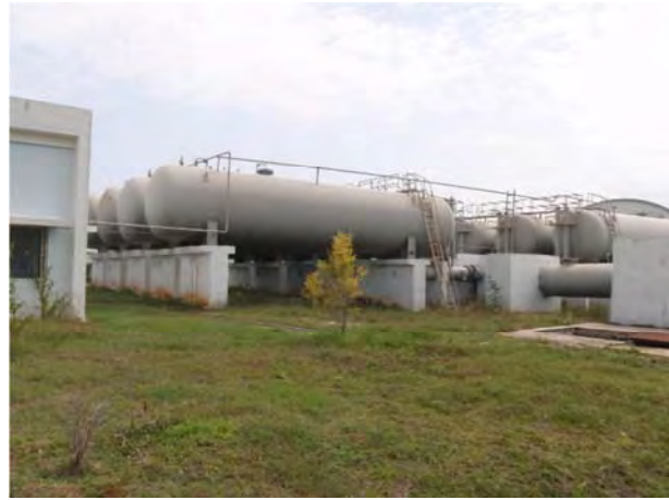
Photo 3.2.4 Air Chamber at TK Halli WTP
