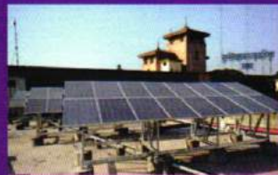
Solar power over PMC building
