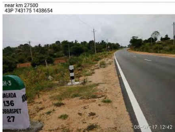
Existing road condition of SH-3 (Km Ch. 27.500)
