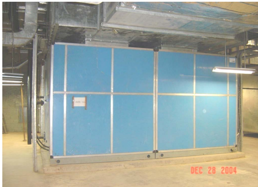
Concourse Air Handling Unit
