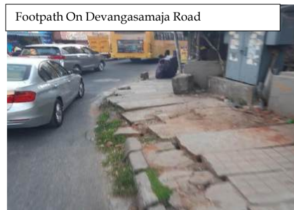
Figure 150. Condition of Footpath Along The Corridor
