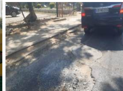
Damaged Road Surface near Baiyappanahalli
