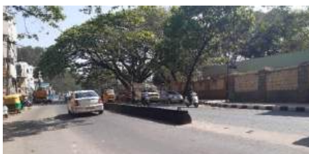
Median End Treatment not done
