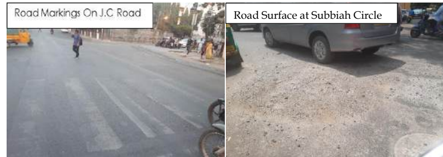
Figure 149. Condition of Road Surface & Road Marking Along The Corridor
