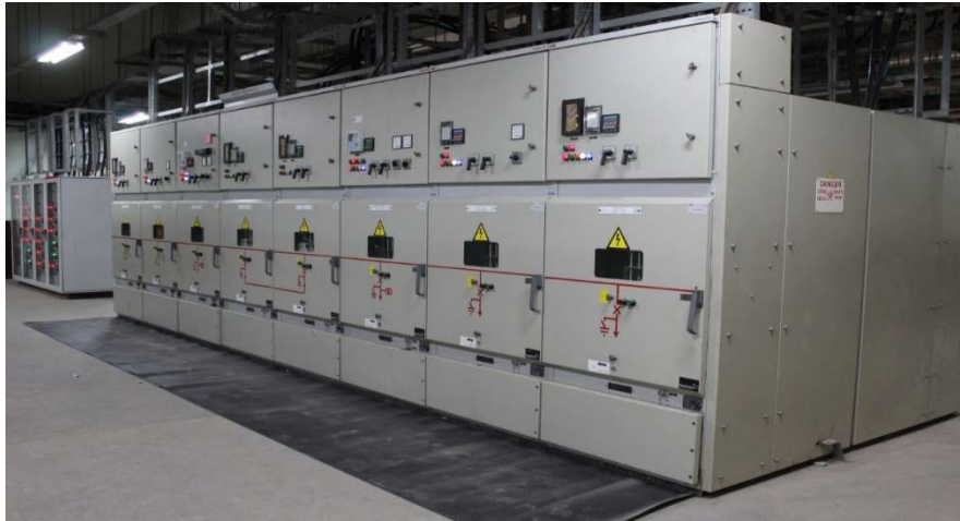
Figure 12.4 Typical Indoor Auxiliary Sub-station
