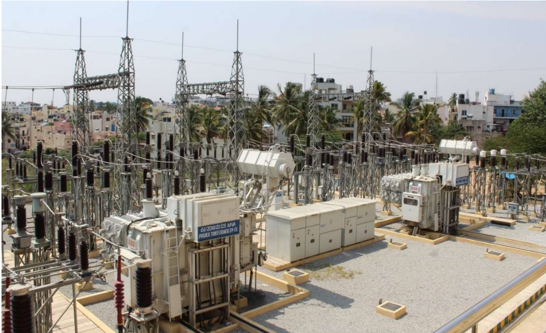
Figure 12.1: Typical High Voltage Receiving Sub-Station
