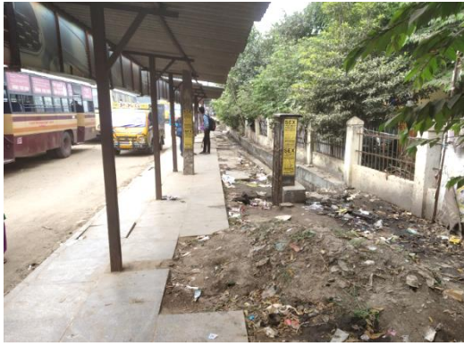
1. Neglected Footpath Facility
