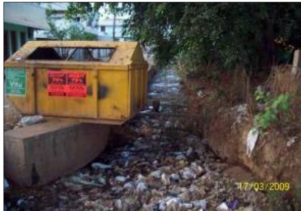
DRAIN NO : DH 368 CHAINAGE :400.0M LOCATION : Near Herohalli Kere Large quantity of garbage dump observed inside SWD
