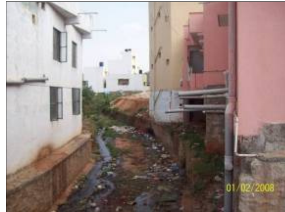
DRAIN NO: RN562A (RNR03), CHAINAGE: 150 m LOCATION: 8 th Cross Main, Jnana Ganga Nagara Water stagnation in the main drain at the outlet Building constructed over the main drain location
