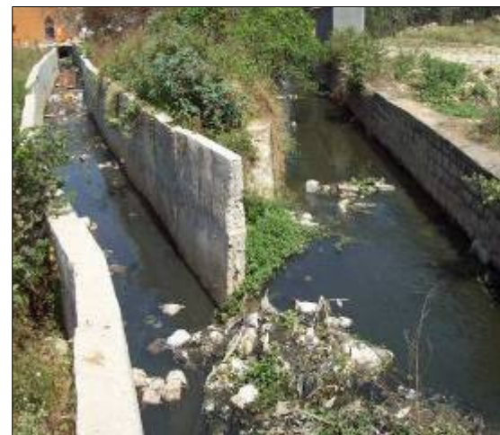
DRAIN NO:MD334 CHAINAGE:620.0M LOCATION: Kalappa Layout Primary and secondary drains are joining at same bed level. Vegetation growth observed
