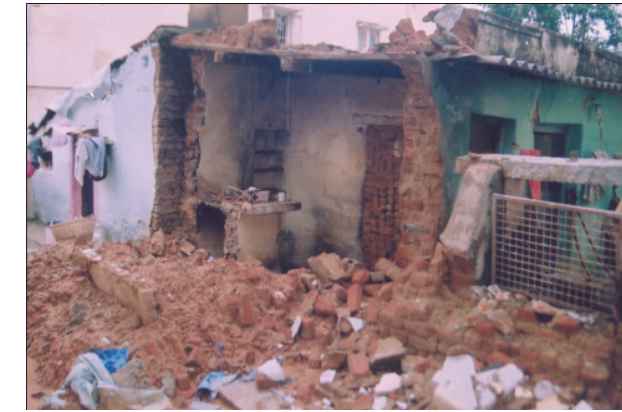
Residential building wall collapsed due to surcharging of water during heavy rains in the SWD
