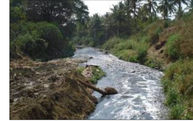
DRAIN NO. RN181 CHAINAGE :8925.0M LOCATION :Near Swami Narayana Gurukula Ashram Drain reach is in natural condition, large quantity of sewage flow is observed, dumped debris obstructing flow of water.
