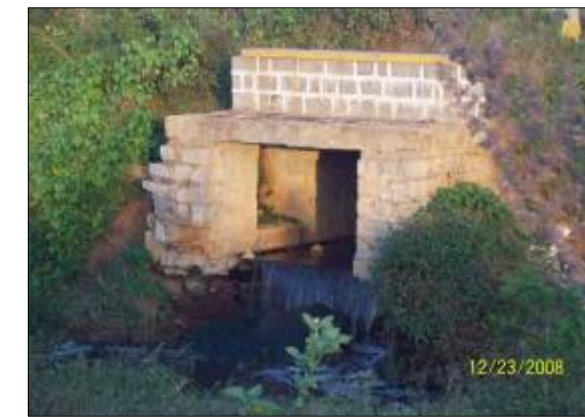
DRAIN NO. RN 541 CHAINAGE : 2000.0M LOCATION :Vishveswaraya layout Due to non existence of sewer network,Raw sewage flow observed in SWD
