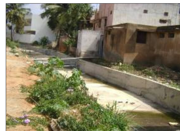
LLA ID: MDLA084 LOCATION : Near Ashrama Road Sanitary and water pipe lines laid across SWD on upstream side
