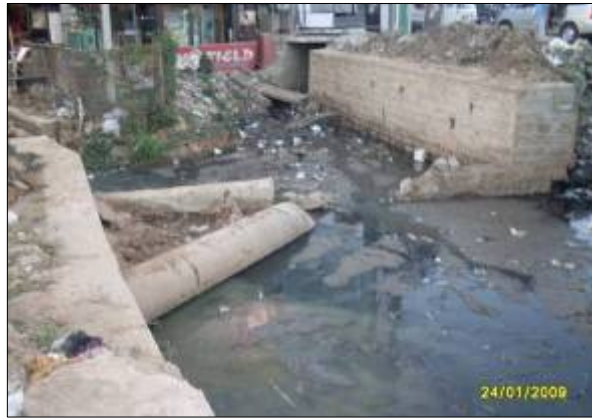
DRAIN NO. BP176 CHAINAGE :1225.0M LOCATION: Sahakara nagara (LHS of Bellary road) Disused RCC pipes lying inside SWD and severely Silted
