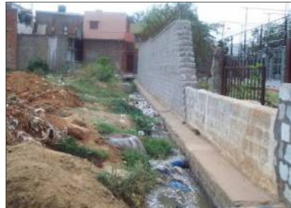
DRAIN NO. BH614 CHAINAGE: 525.0M LOCATION: Parappana Agrahara Drain reach is in natural condition width Reduced, alignment modified, Manhole exists
