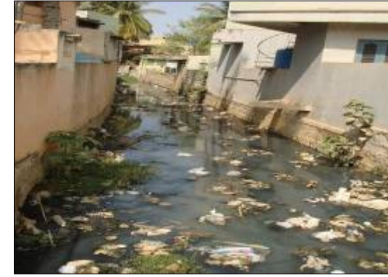
DRAIN NO : MD264 CHAINAGE :1100.0M LOCATION : Ramamurthy Nagar Due to insufficient bed gradient sewage flow observed in the drain
