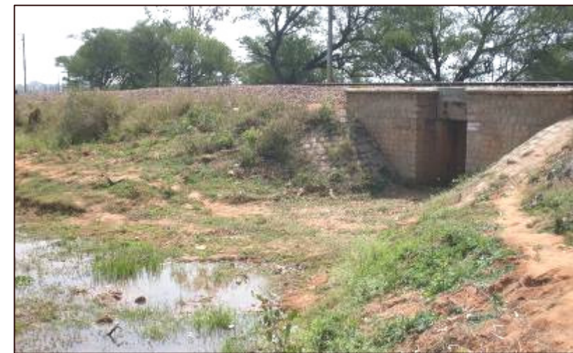
Railway Culvert having inadequate vent way constructed across Storm Water Drain in Yelahanka Zone is causing obstruction for free flow of water
