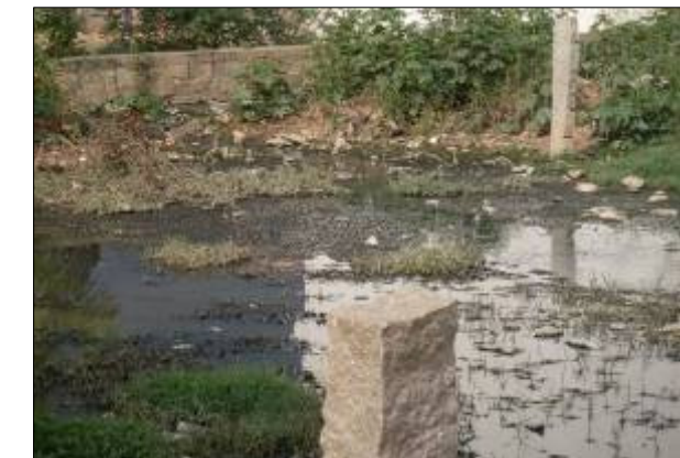
DRAIN NO. BH614A CHAINAGE :360.0M LOCATION :Near G.K Layout Drain reach is in natural condition severely silted sewage stagnation observed
