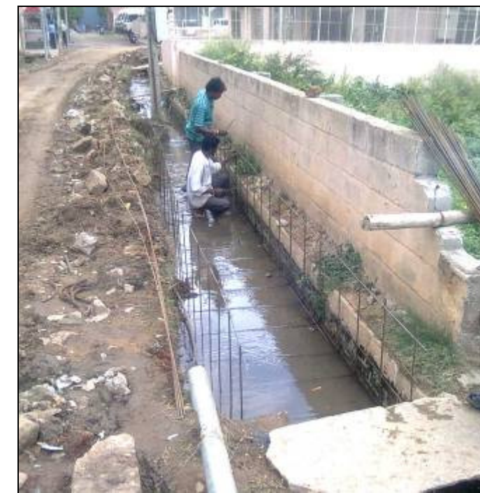
Tertiary / road side drain wall construction at low lying area in RR nagara
