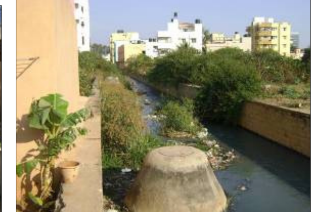
LLA ID: MDLA114 LOCATION : Near Abaya Reddy Layout, Vijnana Nagar Large quantity of vegetation growth observed inside SWD Manhole laid inside the drain
