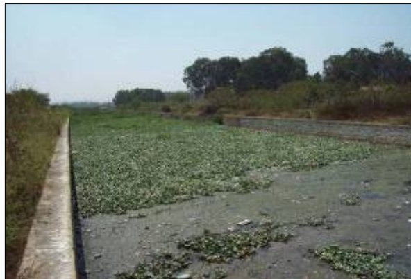
DRAIN NO. MD349 CHAINAGE :200.0M LOCATION : Near Panathur-Varthur Road Due to insufficient bed gradient large quantity of Sewage stagnation and weed growth observed
