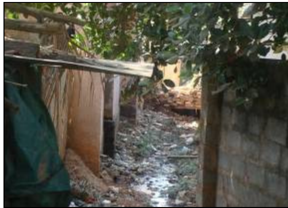
DRAIN NO: MD423 CHAINAGE:0.0M LOCATION: Ramagondanahalli Drain reach is in natural condition, vegetation growth observed, buildings constructed inside waterway
