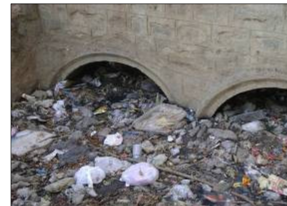
LLA ID. MDLA089 LOCATION : Nethravathy Layout RCC hume pipe laid across SWD is completely blocked and water stagnation Observed due dumping of garbage inside swd
