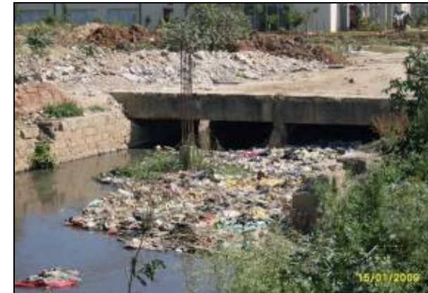
BP183, Ch. 700 m. near Manyatha Tech Park, Mariyyanapalya Accumulation of solid waste materials inside the SWD
