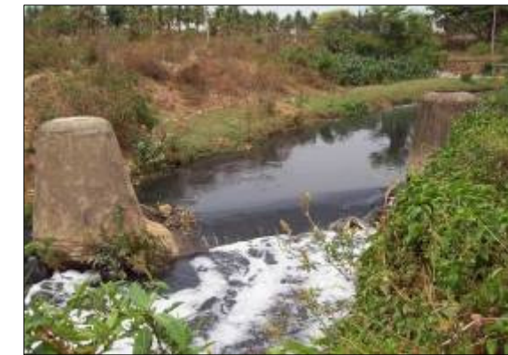
DRAIN NO. RN223 CHAINAGE :8225.0M LOCATION: BEML Layout Trunk sewer pipeline is laid across SWD, i.e., exactly on bedline is obstructing free flow of water in turn causing water stagnation on upstream side
