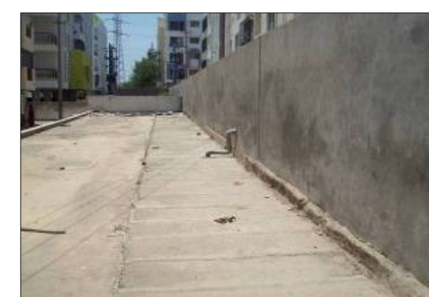
DRAIN NO. MD313 CHAINAGE: 250.0 M LOCATION: Kaggadasapura Drain reach is covered with RCC slab by Apartment developers, width reduced
