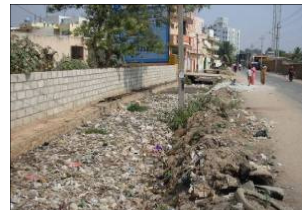
DRAIN NO. BH578 CHAINAGE :800.0M LOCATION : Near Muniyappa Layout Drain reach is in natural condition, large quantity of garbage observed and road level and drain invert level are in same level
