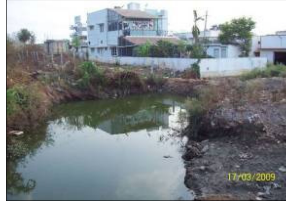
DRAIN NO : DH 370 CHAINAGE :1025.0M LOCATION : Hoysalanagara Original alignment modified, drain reach is in natural condition, sewage stagnation is observed, building constructed inside water way
