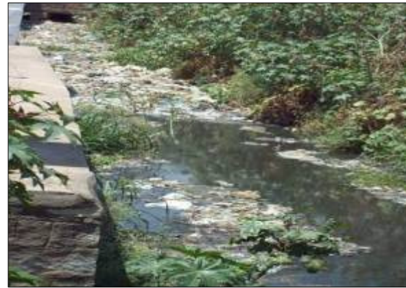
DRAIN NO. BH577 CHAINAGE :25.0M LOCATION: Near Hongasandra Drain reach is in natural condition large quantity of sewage stagnation observed
