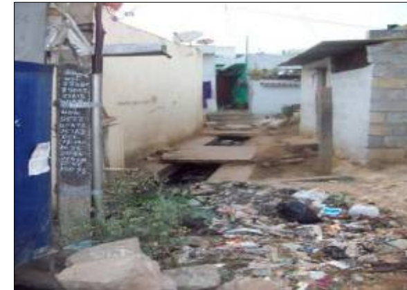
DRAIN NO. BH614 CHAINAGE: 130.0M LOCATION: Parappana Agrahara Drain width is drastically reduced, building constructed inside the water way
