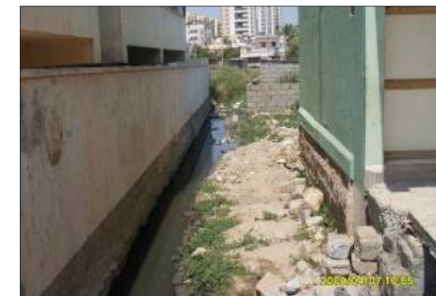
DRAIN NO. BH528 CHAINAGE :1500.0M LOCATION :Near Hulimavu Kere Original alignment modified, waterway encroached building constructed inside waterway
