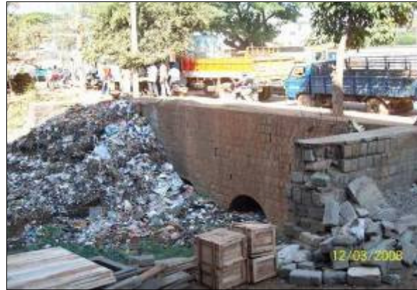
DRAIN NO. DH 211,211A & B CHAINAGE :725.0M LOCATION : Near TVS Cross Large quantity of garbage dumped over culvert Location
