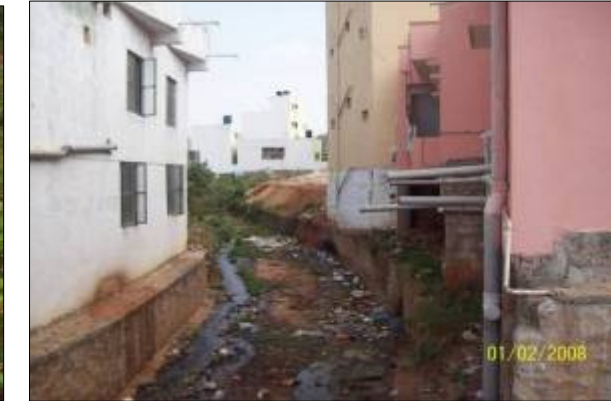
DRAIN NO. RN562A(RNR03) CHAINAGE150M LOCATION : Jnana Ganga nagara Buildings constructed upto the edge of the drain wall, sewer outlets from residential buildings directly connected to SWD
