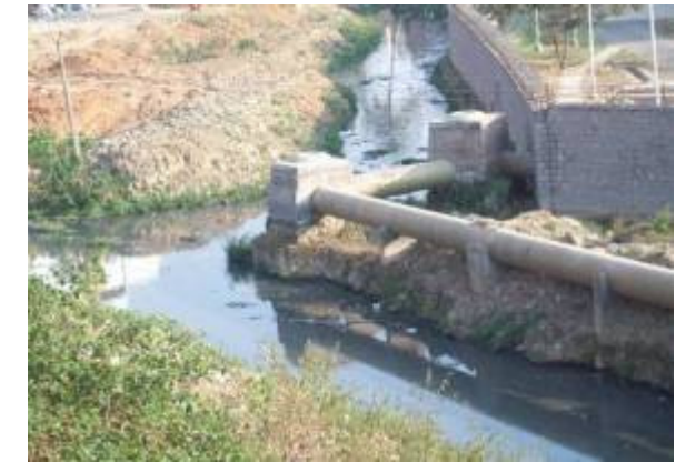
DRAIN NO. MD312 CHAINAGE : 975.0M LOCATION : Nagara Palya, Benniganahalli HDPE pipeline laid inside waterway above bedlevel.
