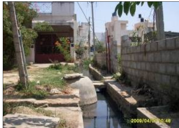
DRAIN NO. BH528 CHAINAGE: 1400.0M LOCATION: Near Kammanahalli Main Road Manhole constructed inside waterway is Obstructing free flow of water
