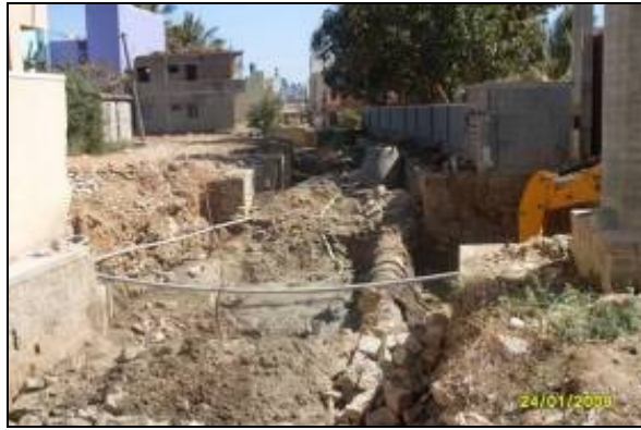
DRAIN NO. BP161 (BY013) CHAINAGE :420.0 M LOCATION : Near Yelahanka New town Bus stand Sewer pipeline laying work inside SWD in progress debris dumped on wet bed, pipeline with manhole running longitudinally
