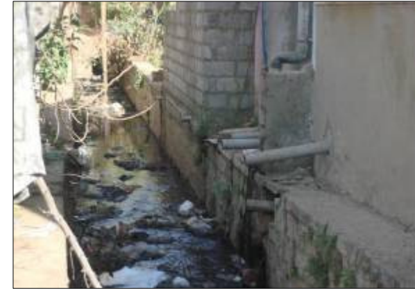
DRAIN NO:MD331 CHAINAGE:675.0M LOCATION: Near Vibuthipura Kere Sewer outlet from residences directly Connected to SWD
