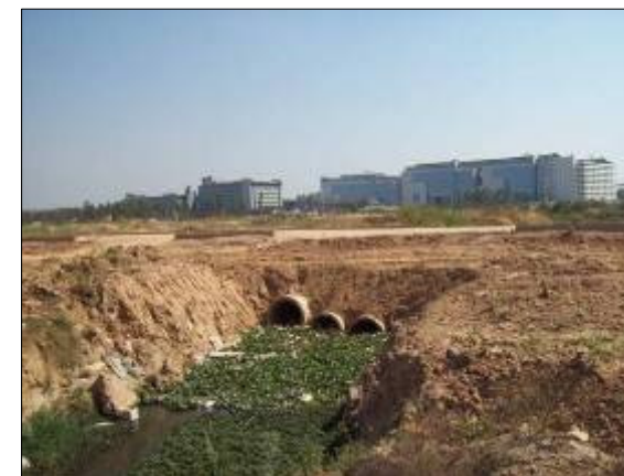
DRAIN NO. MD349 CHAINAGE :2350.0M LOCATION :Near Marathalli Main Road Original alignment modified, width drastically Reduced.
