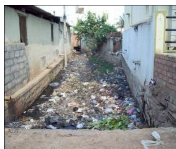
DRAIN NO. BH576 CHAINAGE :225.0M LOCATION :Near Ambedkar Colony Due to insufficient bed gradient largequantity of sewage stagnation observed
