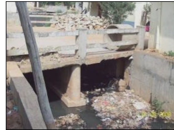
RN562 , Ch.950m 10 th Cross Road, near Bhuvaneshwari nagara Street Sweepings and Floating materials accumulated in SWD
