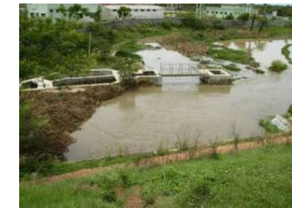
Condition of SWD on upstream side of Rampura Kere, near Raja Canal STP at Zone
