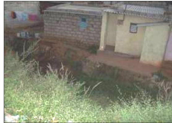
DRAIN NO. RN 553 CHAINAGE: 300.0M LOCATION: Ambedkar Nagar Original alignment modified, drain reach in natural condition, residential buildings constructed inside water way
